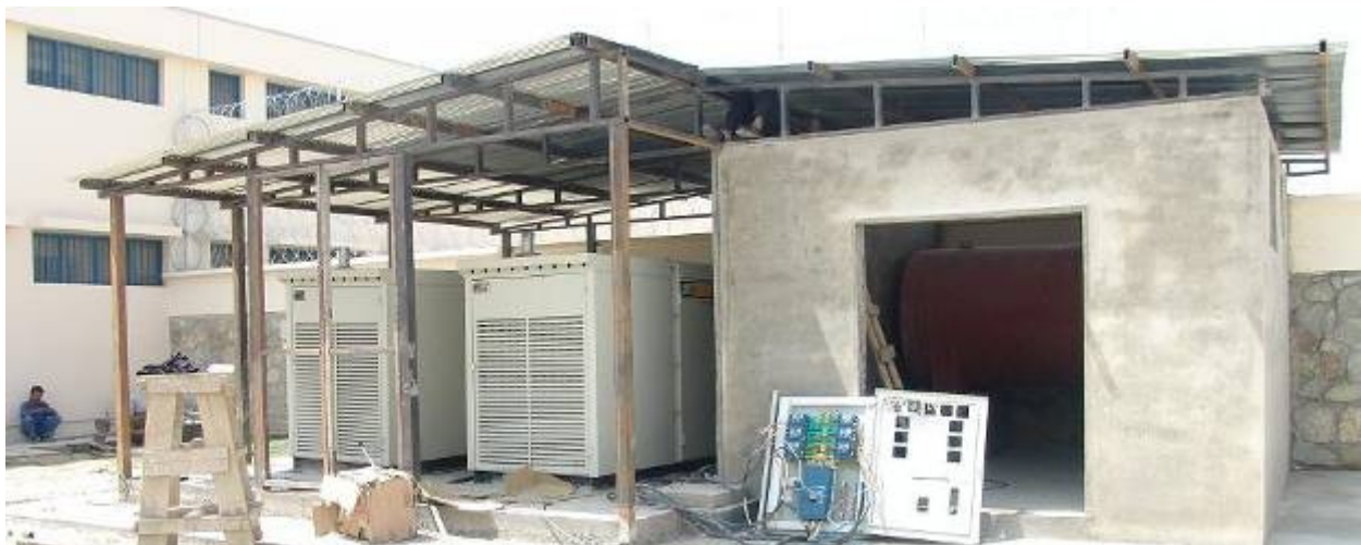
Figure 22 :Generators and fuel store – Expensive to run and install
