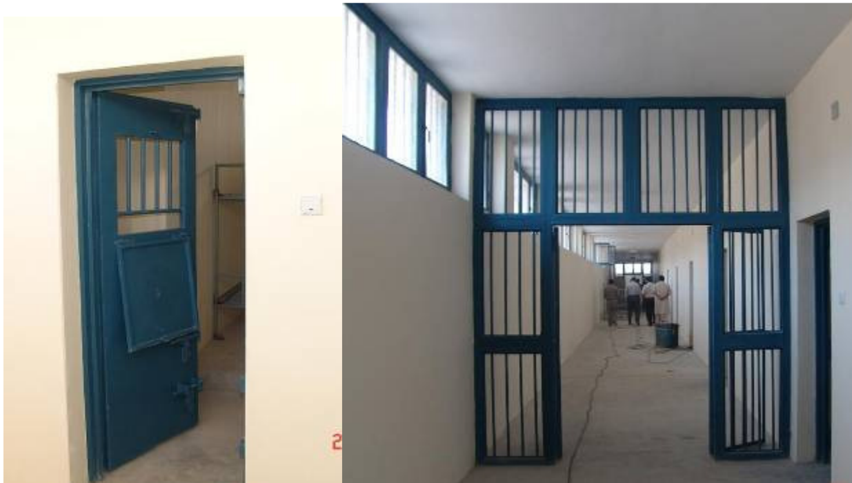
Figure 20 :High security cell door
