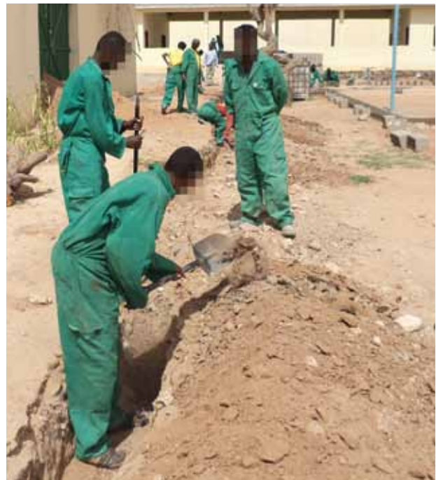
"Trench feat": the inmates dig a trench for a high-voltage cable to their new workshop
