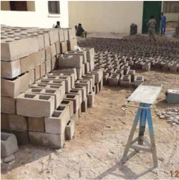
Another brick in the wall: blocks made by inmates provide an additional revenue stream
